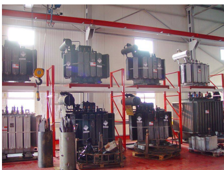
Fig. 1. Temporary storage of high-voltage industrial transformer (source: [9])
