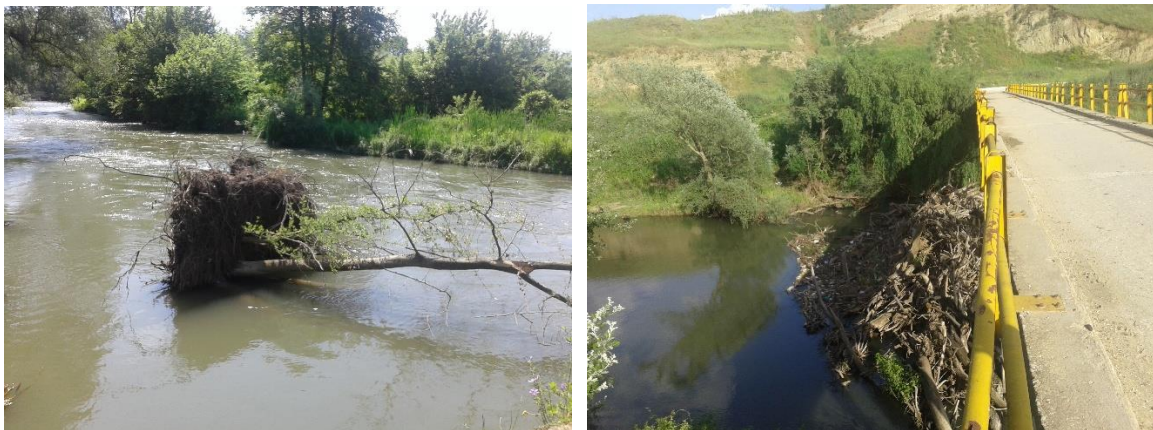
Fig. 2. Tree debris due to soil erosion by high water discharge (left) and debris accumulation at one of the bridges (right).
