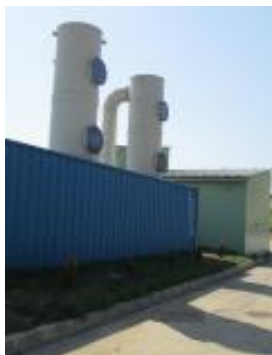
Fig. 1. Overview of the leachate treatment plant
