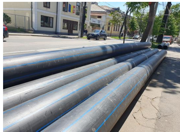
Fig. 5. Polypropylene pipes for the water network
