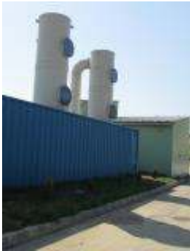
Fig. 1. Overview of the leachate treatment plant
