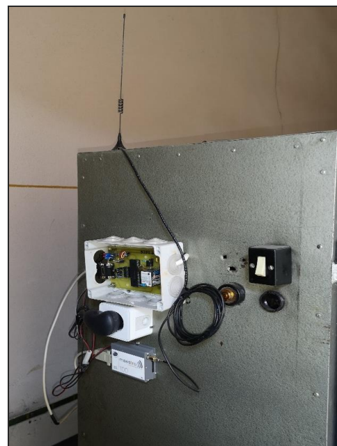
Fig. 7. Switch heating remote control device, mounted on a metal panel
