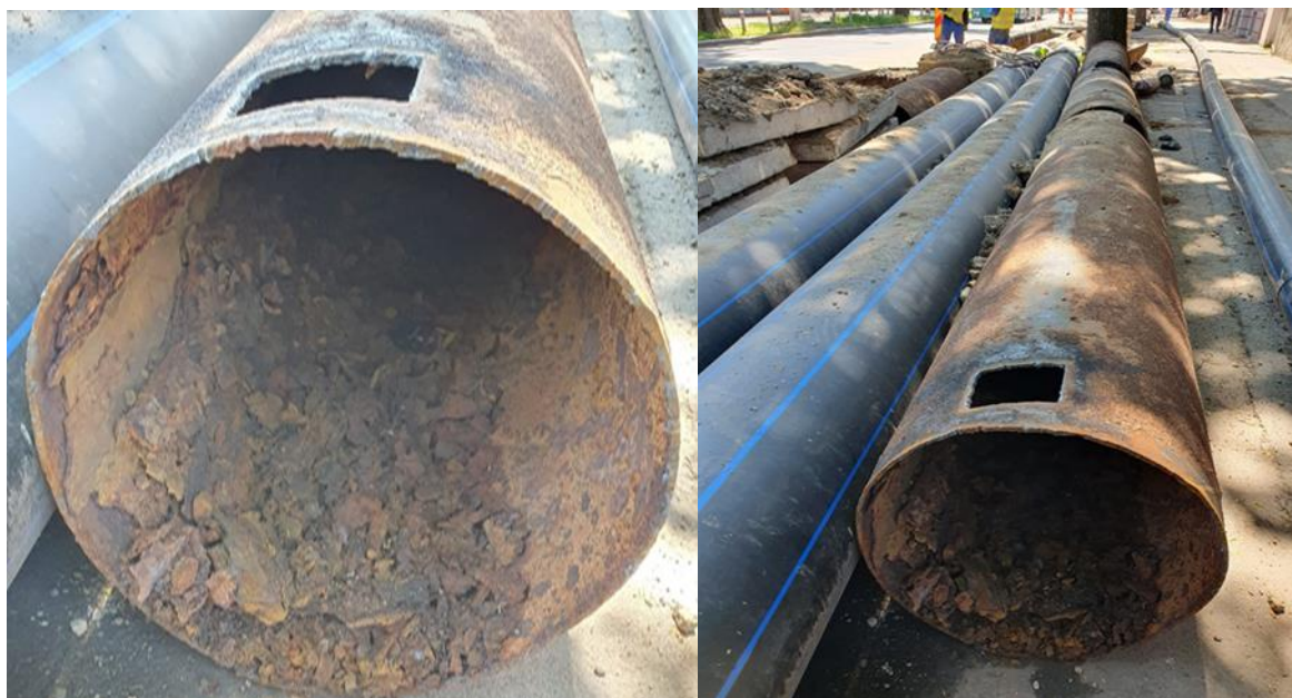
Fig. 1. The pipes with an advanced degree of corrosion and deposits
